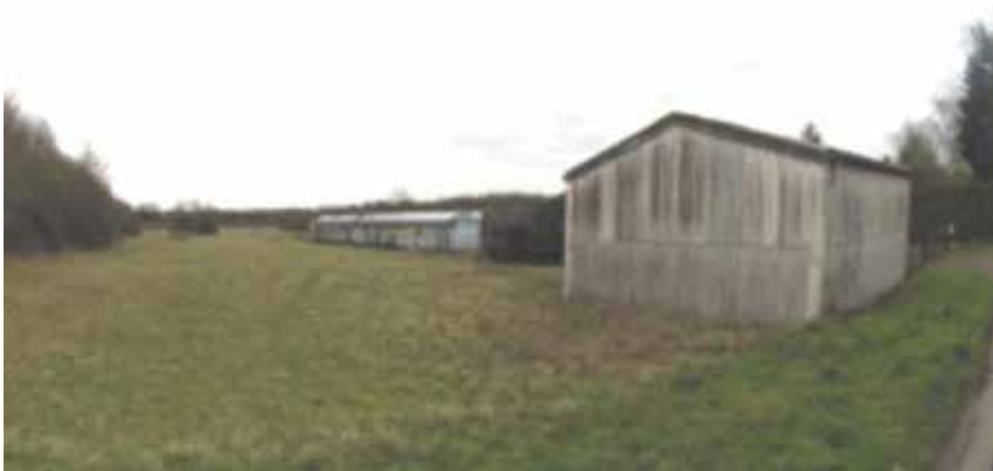
Figure 14: Buildings in poor repair and unused land
